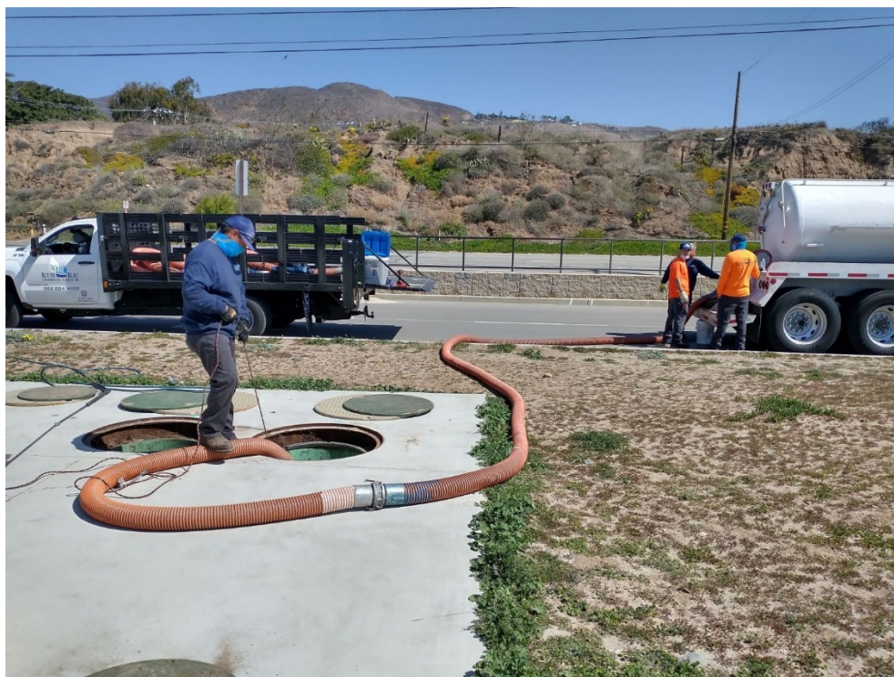
Figure 2-2. Pumping at Zuma Beach Restroom #9 on March 22, 2021.
